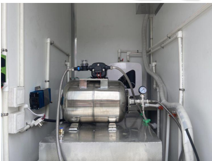
- Water Pressure Tank -
